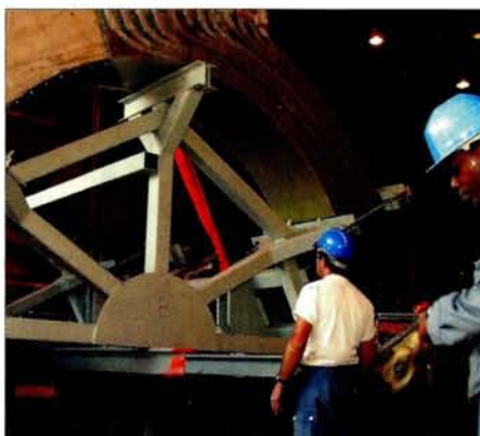
The safe arrival of the coils at CERN.
