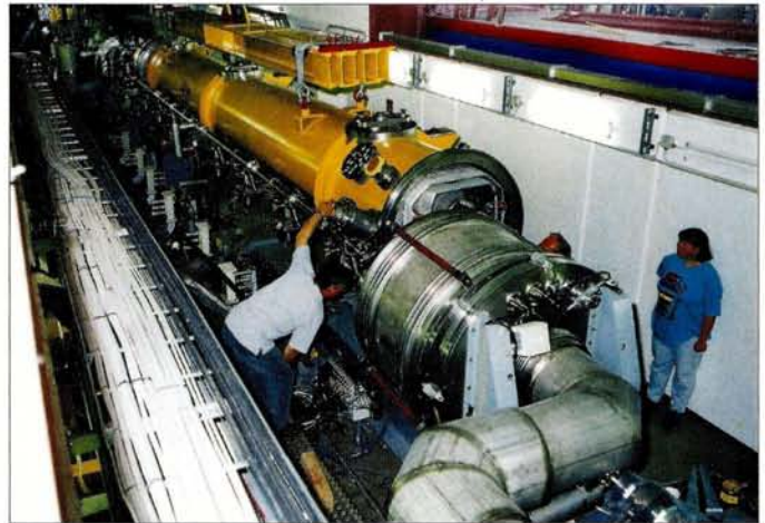
In 2004 the TESLA test facility, which has been extended to reach an energy of 1 GeV, will become available as a user facility for soft X-ray experiments. (DESY Hamburg.)
