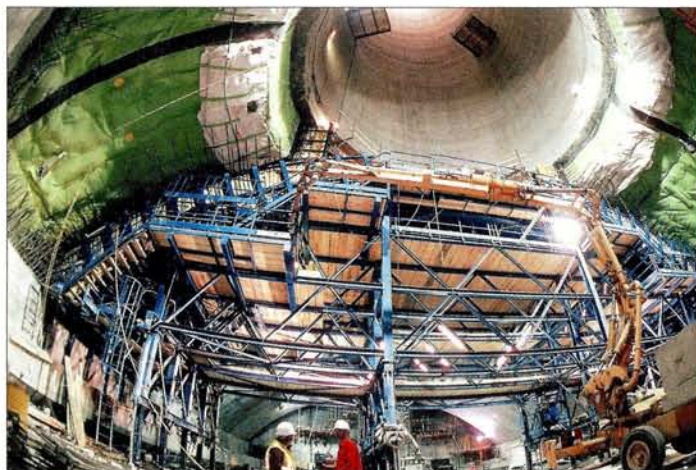
June 2001: the 35 m span for the ATLAS detector hall, UX15, is one of the longest underground spans ever constructed. The ceiling of the 1380 m 2 cavern "hangs" from a system of ground anchors installed from galleries excavated laterally from the access shafts.
