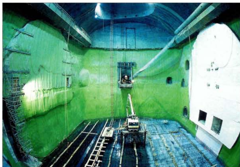
July 2002: the extent of the cavern is clear as the reinforcement of the concrete base is installed.
