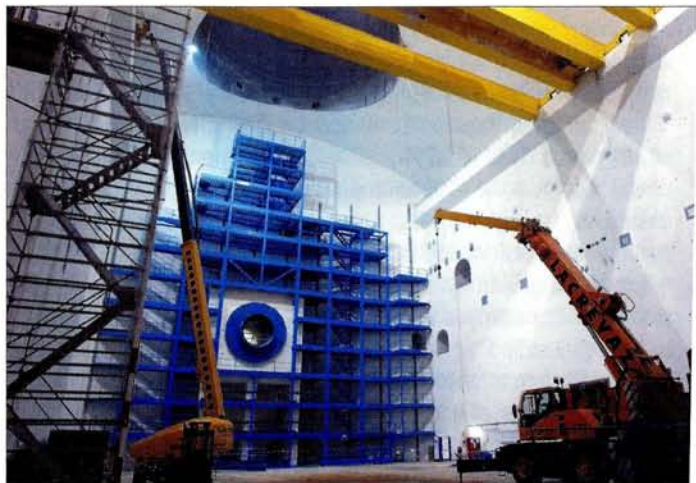
July 2003: a 12 storey metallic structure is one of the first items installed in the completed cavern. Such structures, which will be used for racks of electronics, will surround the detector on all four sides.
